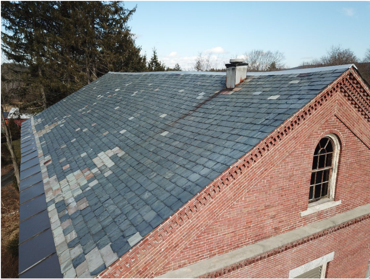
View of natural slate roof and numerous previous repairs with off colored slate. Note: waves in ridge line.
