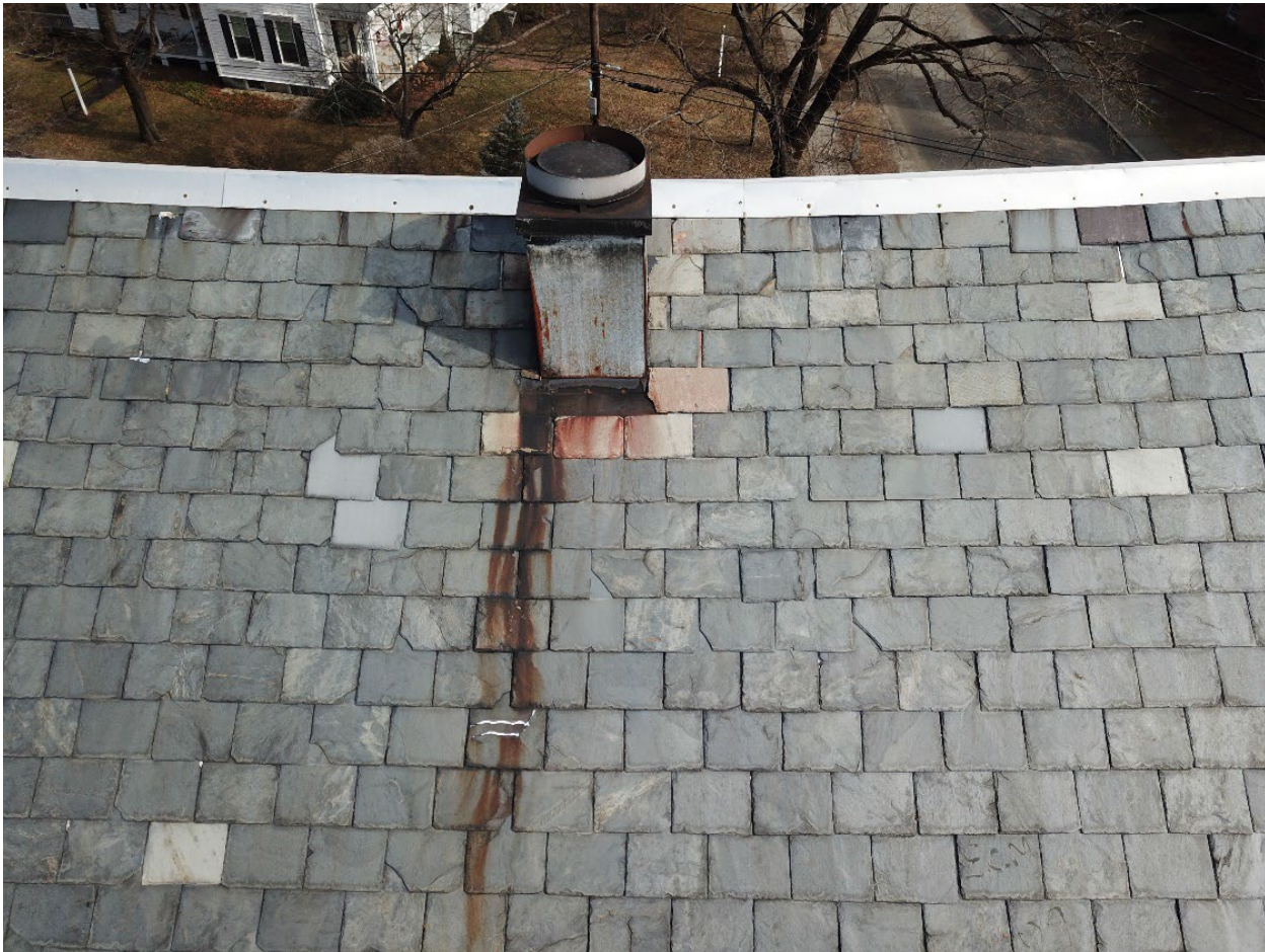
View of roof vent with severe rust at top and bottom flange. Rust is discoloring slate. Ridge cap is face nailed with no washers or sealant visible.
