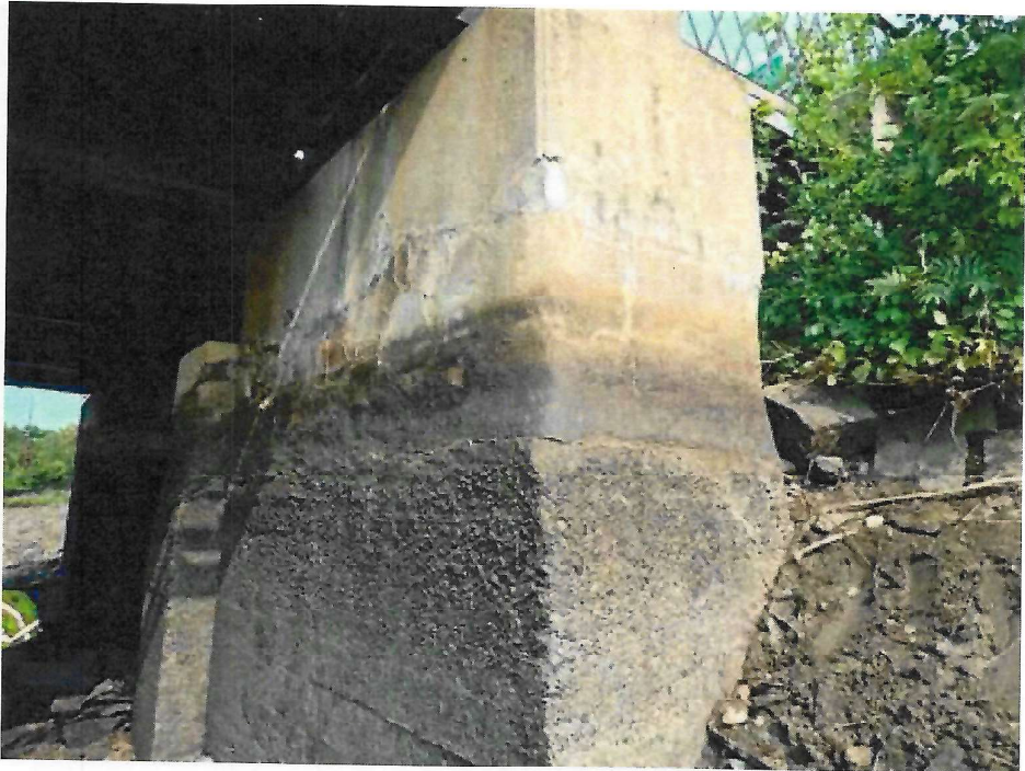
Photo 28: Southeast Pier – abrasion, hollow areas, and cracks around the perimeter at the normal water line
