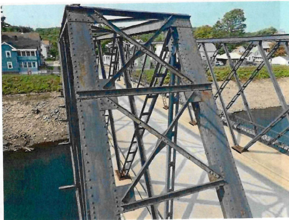
Photo 18: South Truss, at east portal – Web members and bracing with chipped paint with rust
