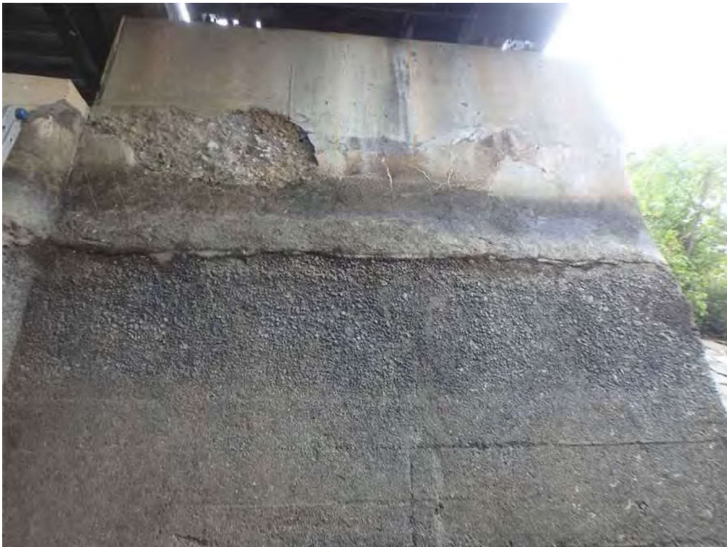
Photo 42: Southeast pier, west face - spall with exposed rebar with an adjacent delamination.
