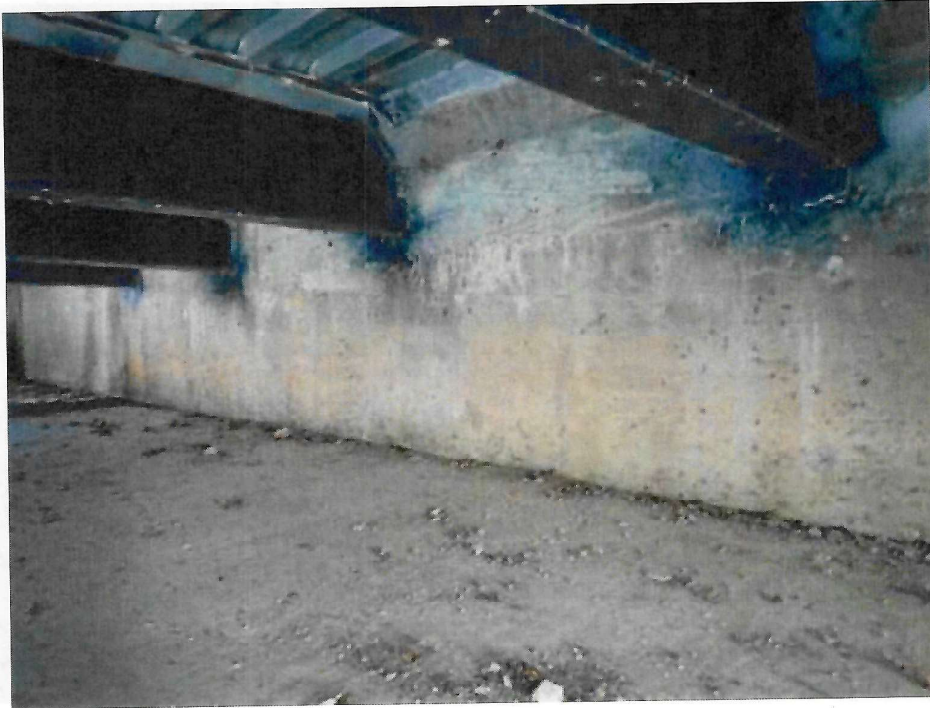
Photo 25: East Breastwall and Backwall with scattered hairline cracks and efflorescence at the stringer ends
