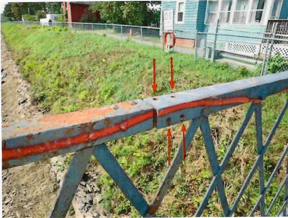
Photo 9: South Pedestrian Railing, at L0, top rail – four (4) missing connection bolts
