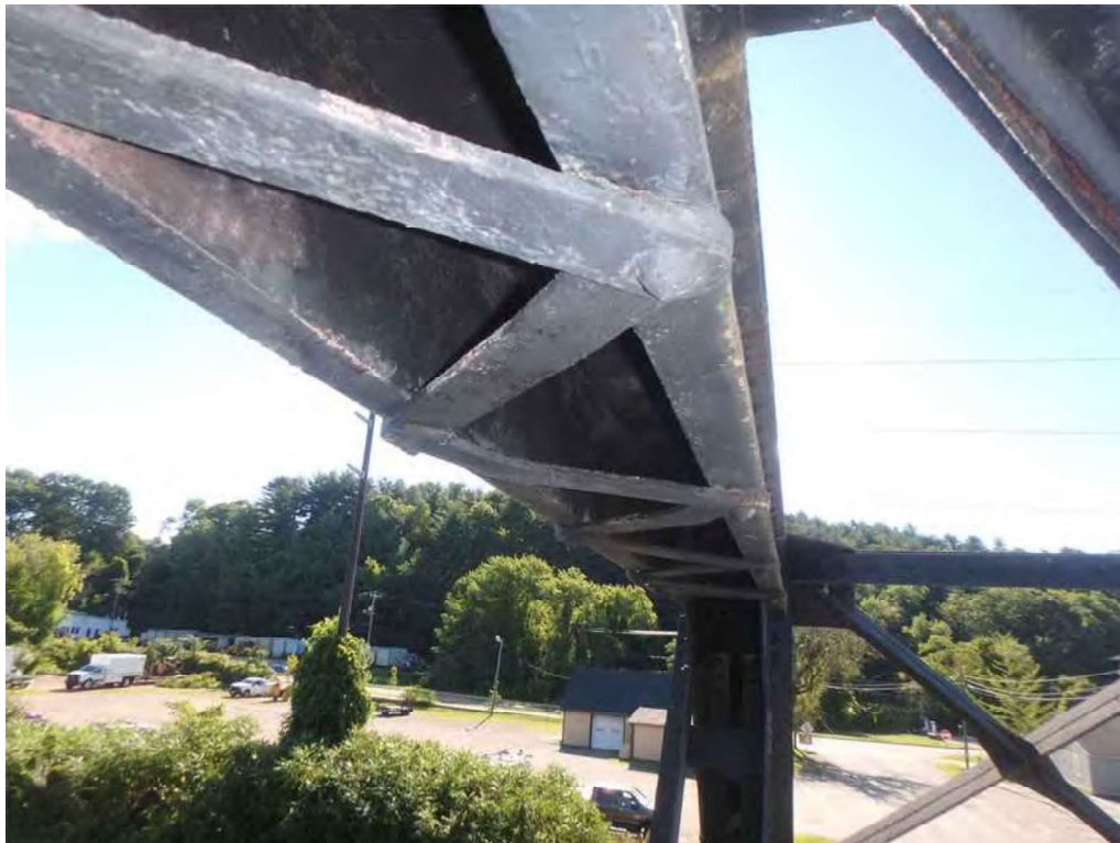
Photo 28: North tower, outer truss, member U14-U16, looking east - bent lattice member.
