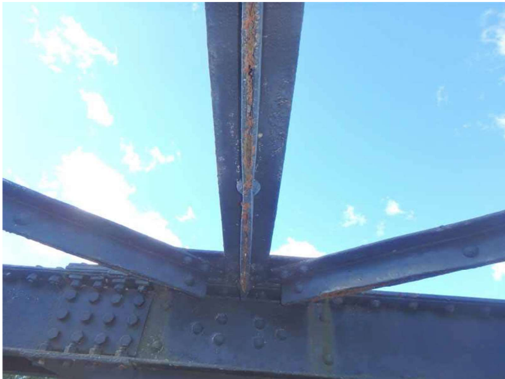
Photo 32: South tower at outer truss, looking south – lateral bracing angles have pack rust between adjacent legs.
