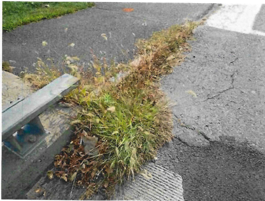
Photo 4: North Curb, East End - Vegetation growth along curb
