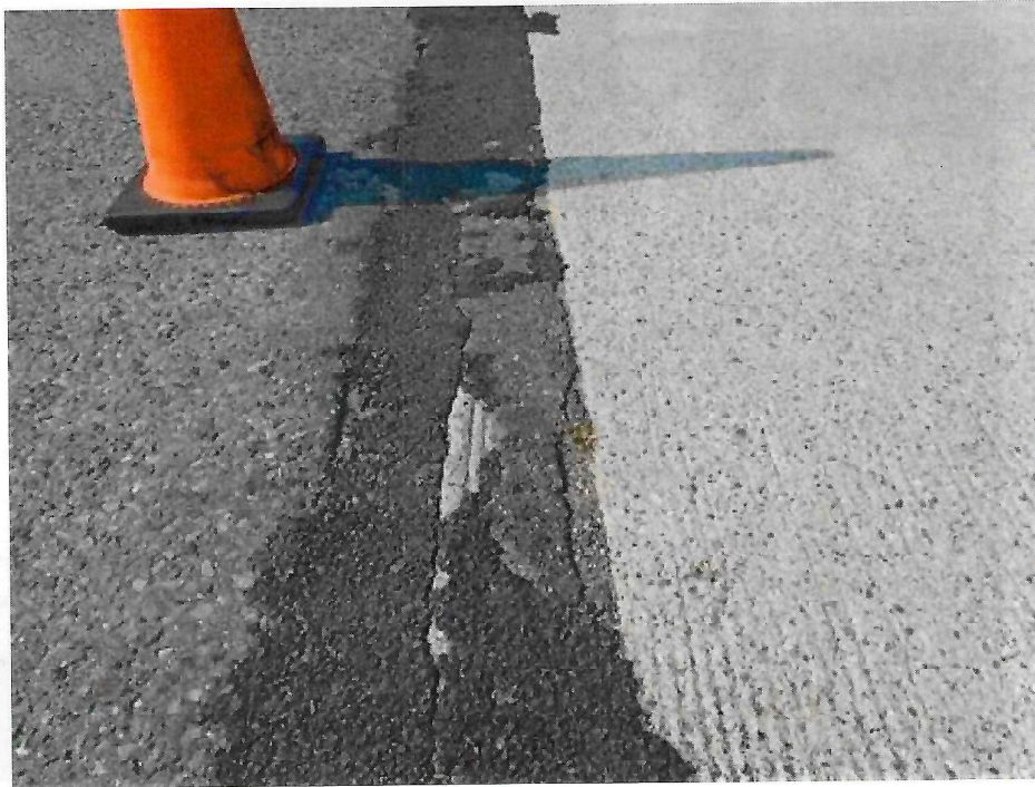
Photo 13: East Abutment and Deck Interface – Bituminous breakup at the middle of the joint
