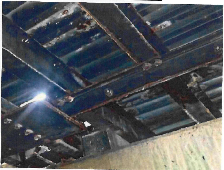
Photo 15: South Sidewalk Stringers, at Southeast Pier – stringers with chipped paint and rust
