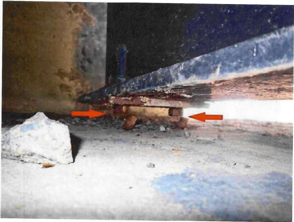
Photo 24: Northwest Pier, at Floorbeam 1 - both anchor rods sheared off. Note the spalled pedestal.
