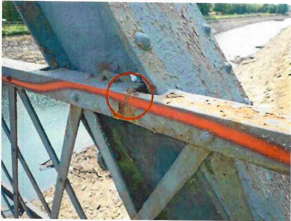
Photo 7: South Sidewalk Pedestrian Railing, top rail, at U1-L0 - crack extending from the cut-out section
