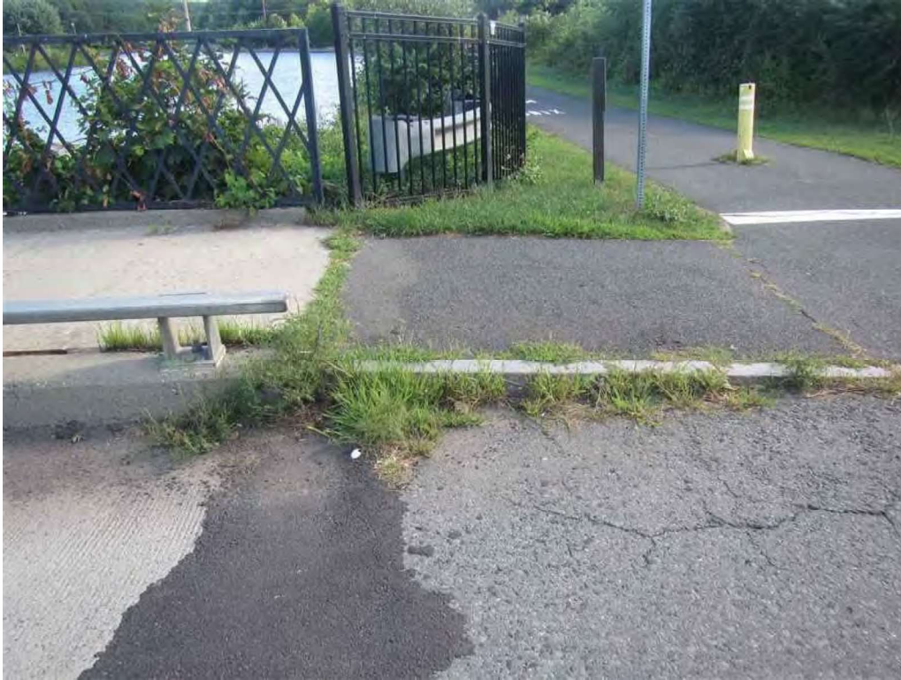
Photo 11: North curb at the east end, at the abutment saw cut - moderate vegetation growth.
