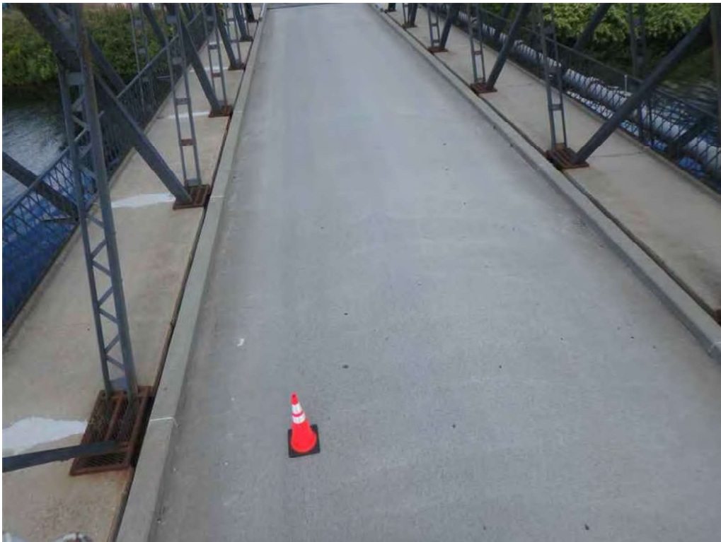
Photo 6: Wearing surface, span 2 shown, looking west - random insignificant cracks.
