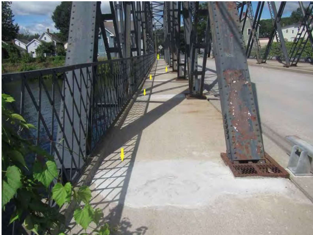
Photo 14: South sidewalk, span 2, at L18, looking west - concrete patch repair at the transverse joints.
