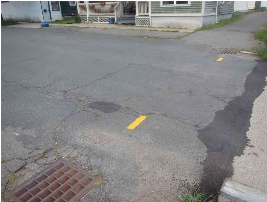
Photo 22: West approach pavement - random longitudinal and transverse cracks. Eastbound lane has a bituminous patch with adjacent area of break-up. Surrounding the drainage basins is bituminous break-up.
