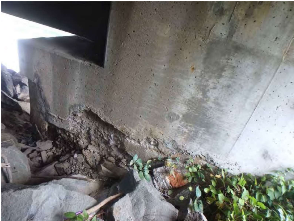
Photo 40: Southwest pier, west face - spall near the base.
