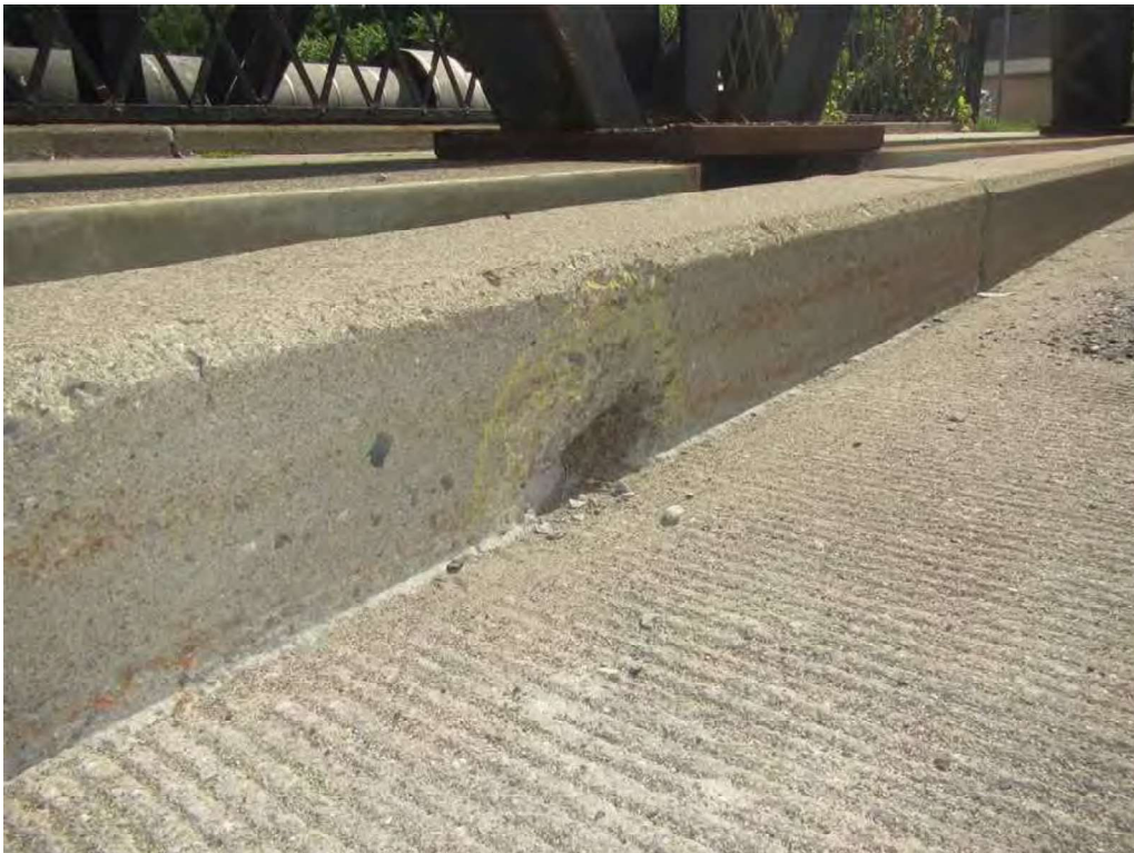
Photo 12: North curb, span 2, near L16, looking northeast - spall.
