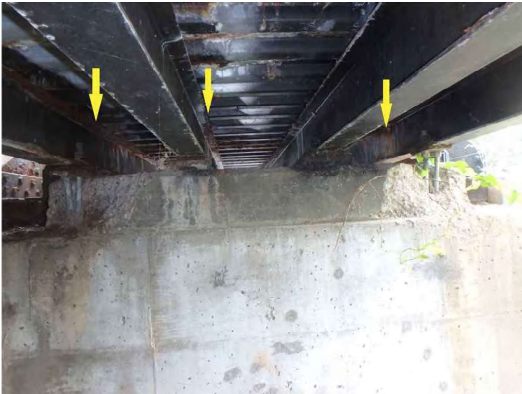
Photo 24: South sidewalk stringers at the southwest pier, looking east - peeling paint and moderate rust. Note the pedestals spalls below sidewalk stringers SW5 and SW8.
