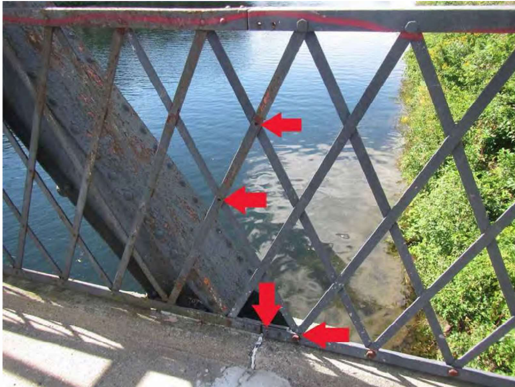
Photo 19: South sidewalk pedestrian railing at L0 - the top and bottom rail splice connections and the lattice members have missing rivets. Additionally, a lattice member to bottom rail connection bolt is loose.
