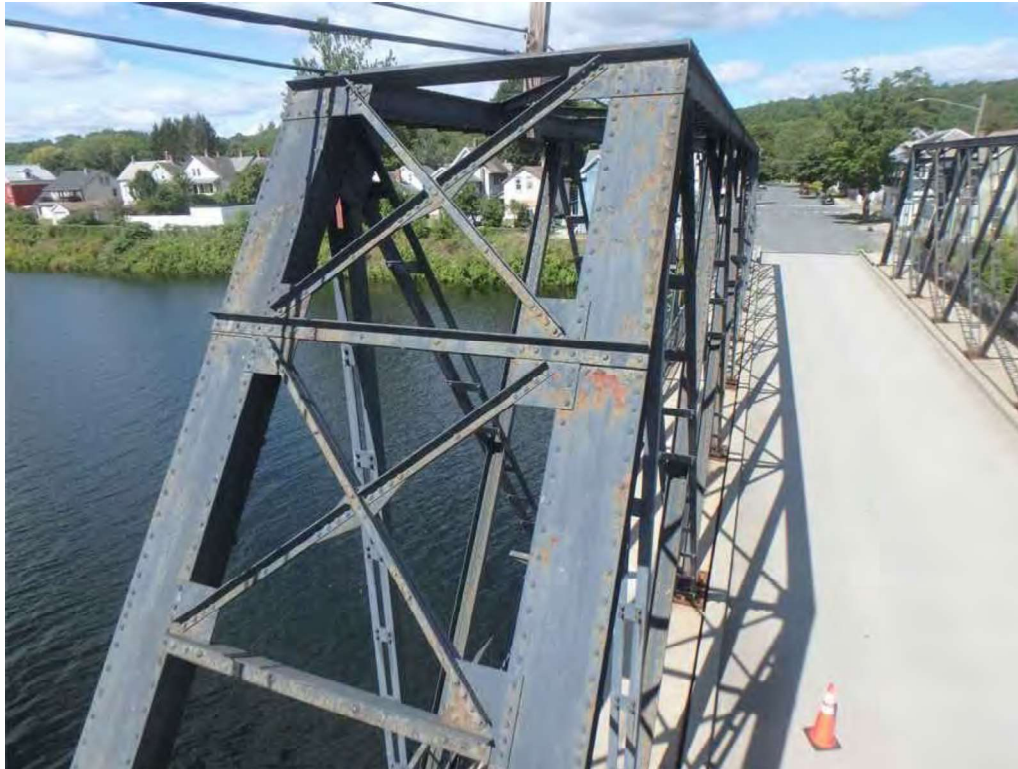
Photo 27: South truss at east portal – end posts and bracing with peeling paint and light rust.
