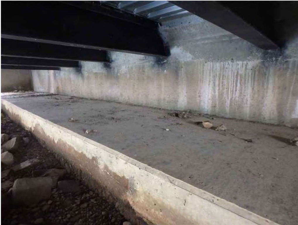
Photo 37: East abutment breastwall and backwall - scattered hairline cracks and efflorescence at the stringer ends.
