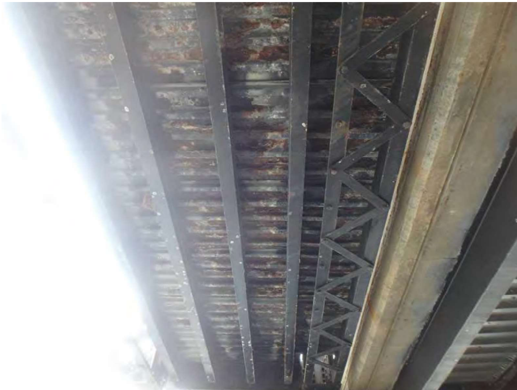
Photo 10: SIP forms, underside of south sidewalk, span 2, panel 9 (between floorbeams 9 and 10), looking west - heavy rust with isolated holes.
