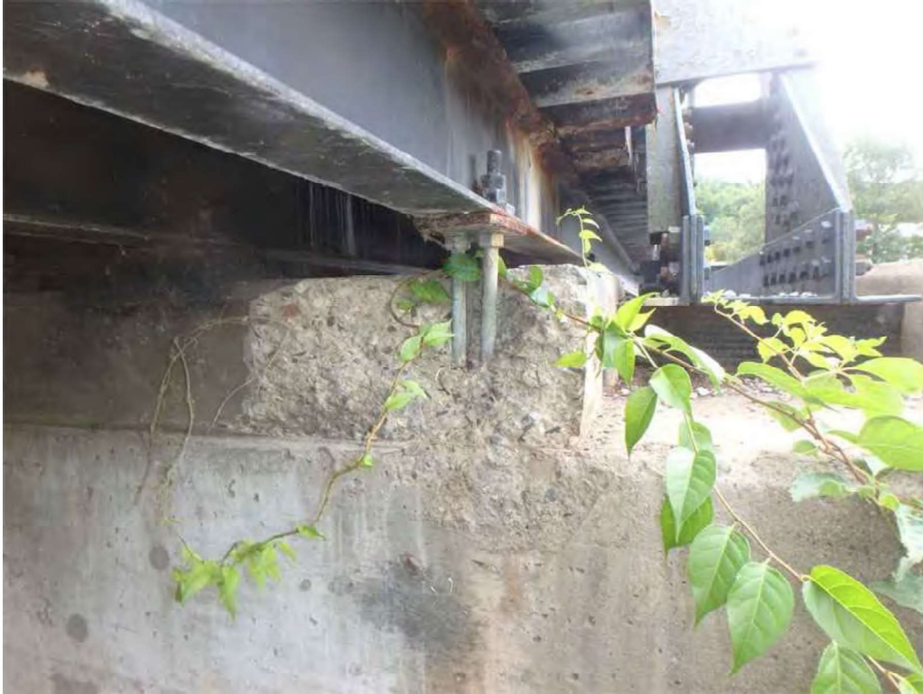
Photo 39: Southwest pier pedestal, west face, at sidewalk stringer SW8 - spall exposing the anchor rods and undermining the masonry plate.
