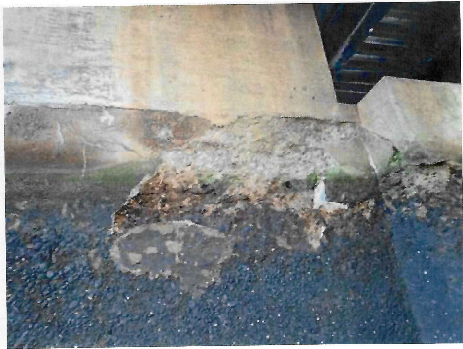
Photo 30: Northeast Pier, West Face, Center – Spall at the normal water line
