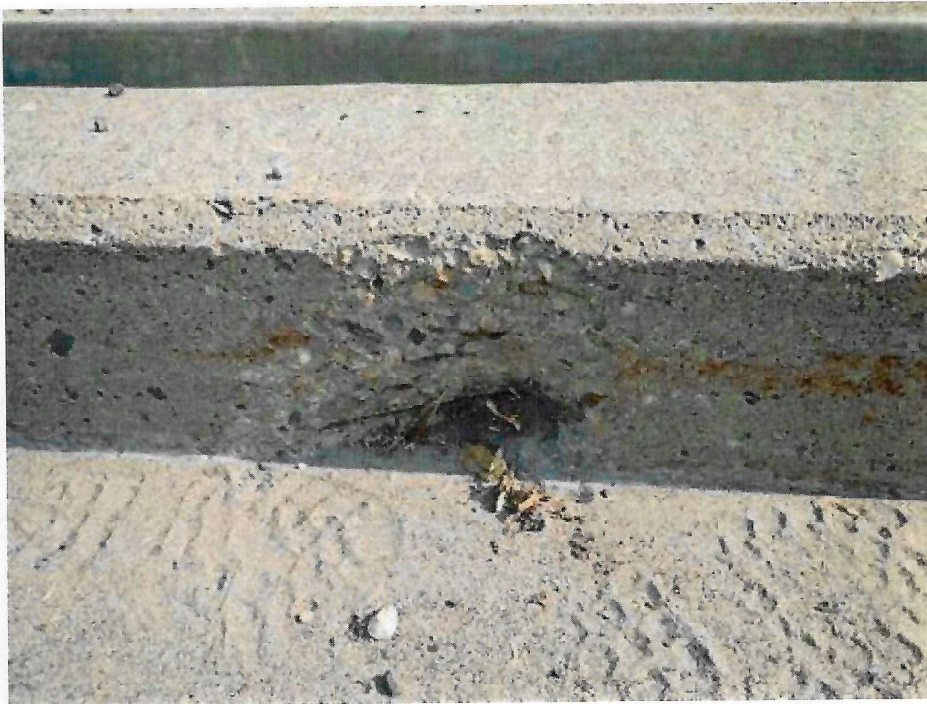
Photo 5: North Curb, near L16 - spall
