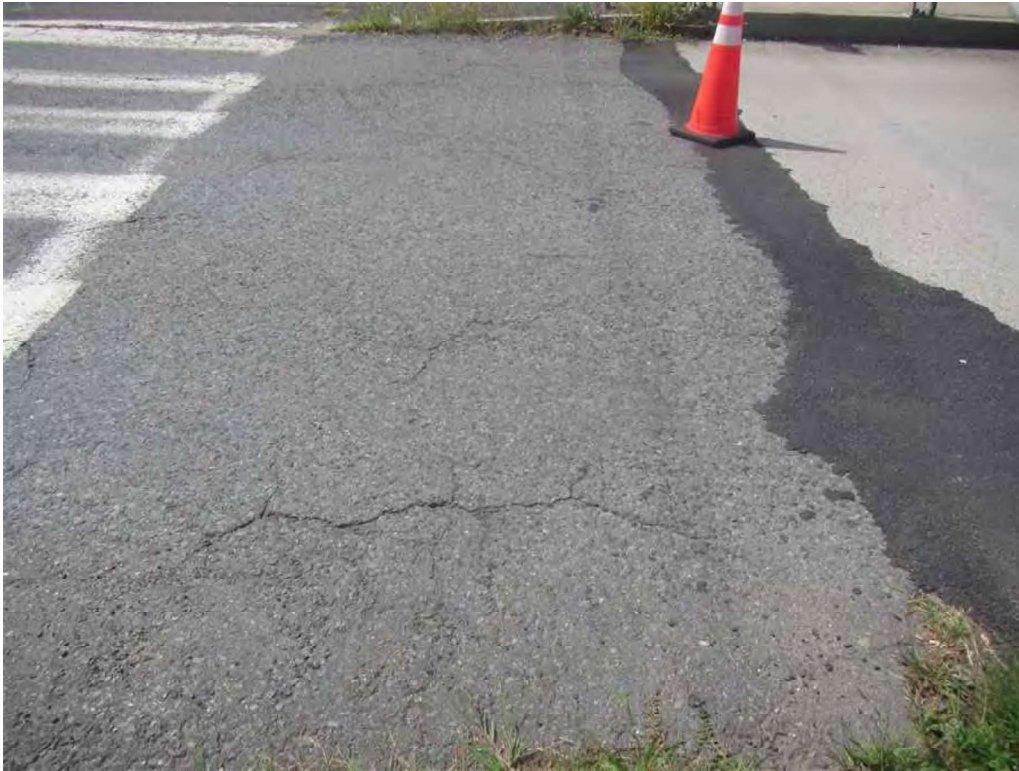
Photo 23: East approach pavement, looking south - random longitudinal cracks.
