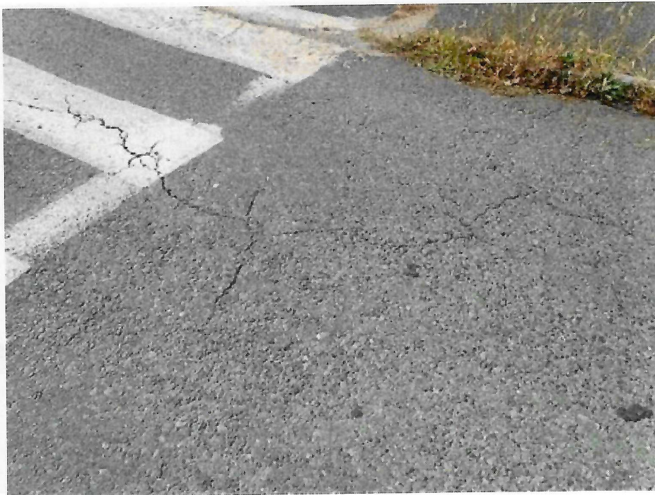
Photo 14: East Approach Wearing Surface - map cracks
