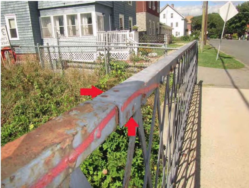
Photo 18: South pedestrian railing at L0: top rail at the splice connection is missing four (4) connection bolts and adjacent sections are laterally misaligned.
