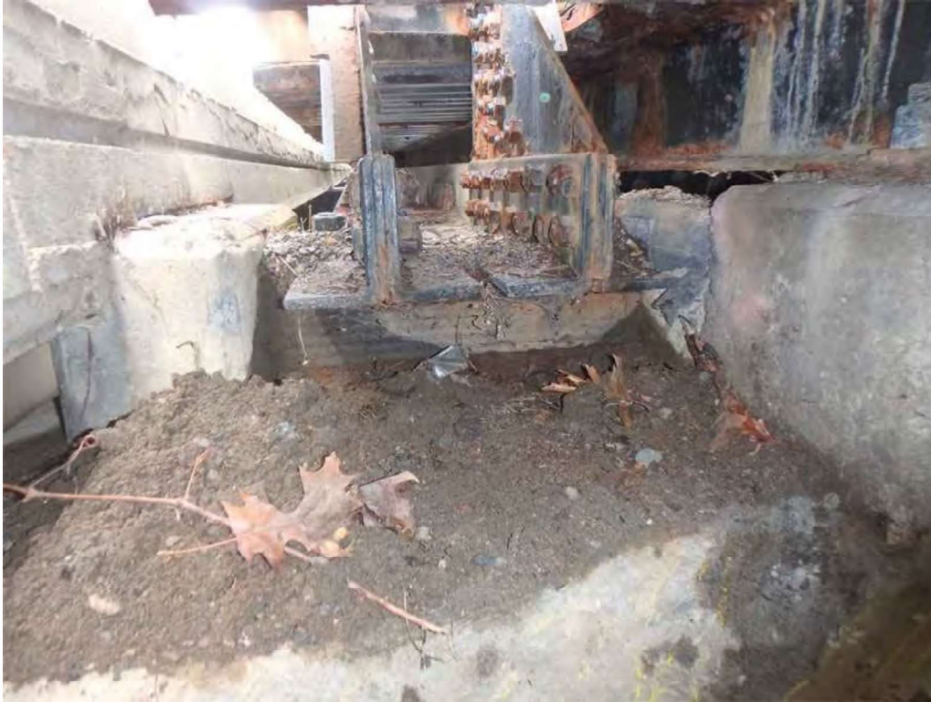
Photo 35: North tower, inner truss, east bearing - steel angles have light to moderate rust and an accumulation of debris that inhibits inspection.
