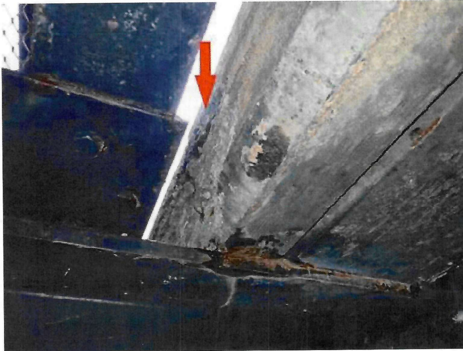
Photo 1: Deck, North Fascia, at FB4 - spall with exposed rebar
