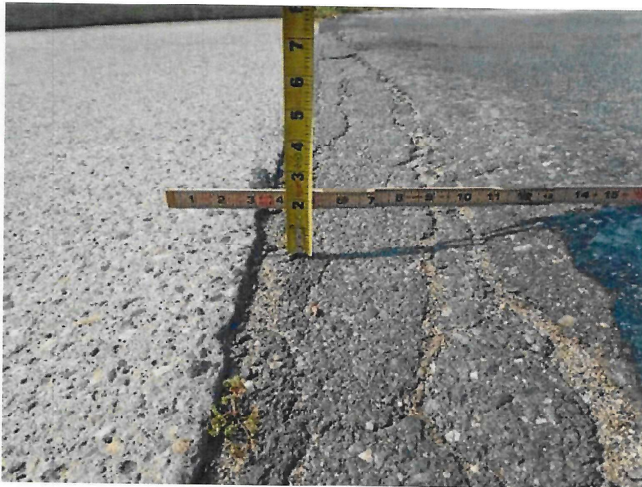
Photo 12: West Abutment and Deck Interface - Bituminous break up and ravelling
