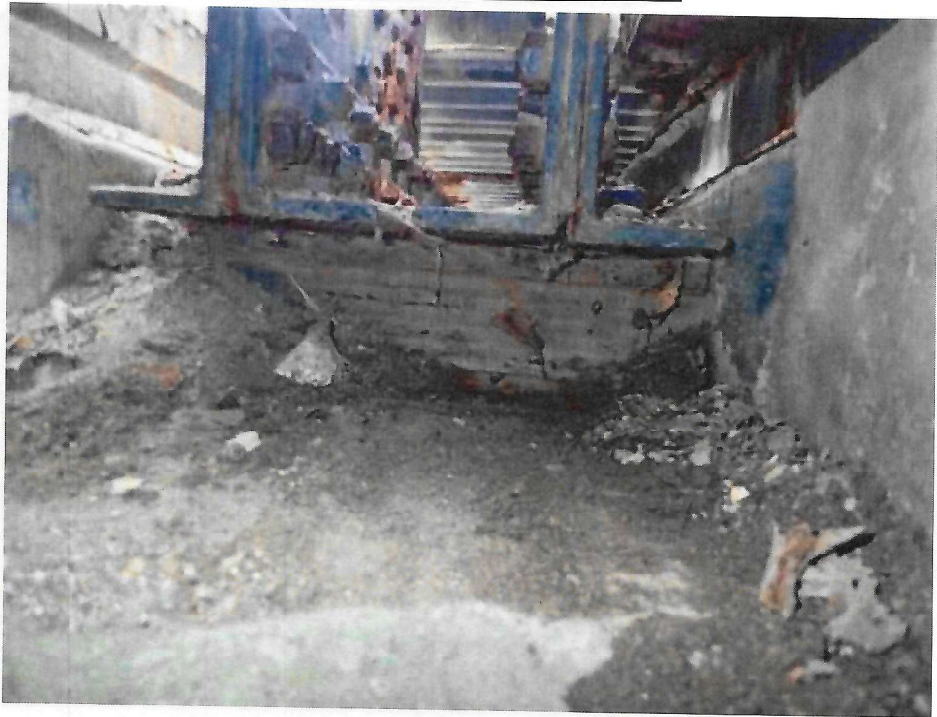
Photo 23: North truss, East bearing with light rust
