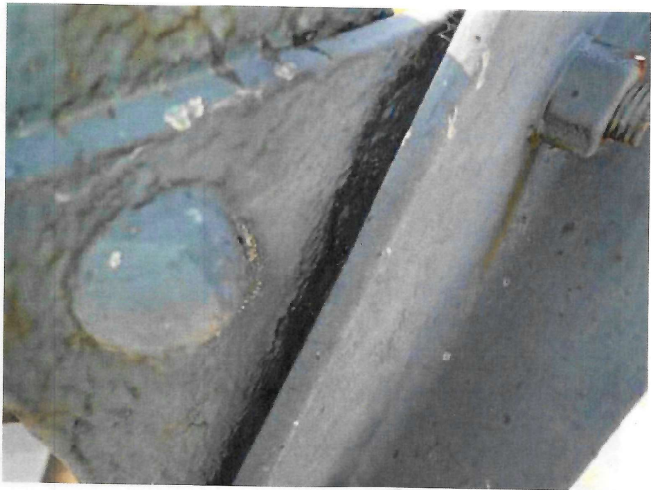
Photo 20: South Outer Truss, U4-L2 at M3 – pack rust and connection plate section loss
