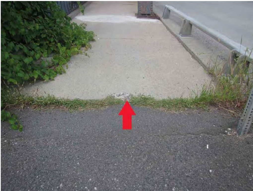
Photo 16: South sidewalk at the east end (at the interface with the southeast approach sidewalk), looking west - edge spall.
