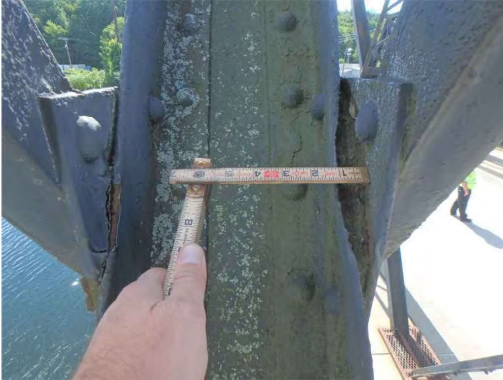
Photo 29: North tower outer truss, member U8-L6 at M7 – the edge of the inner flange has knife edge remaining thickness.
