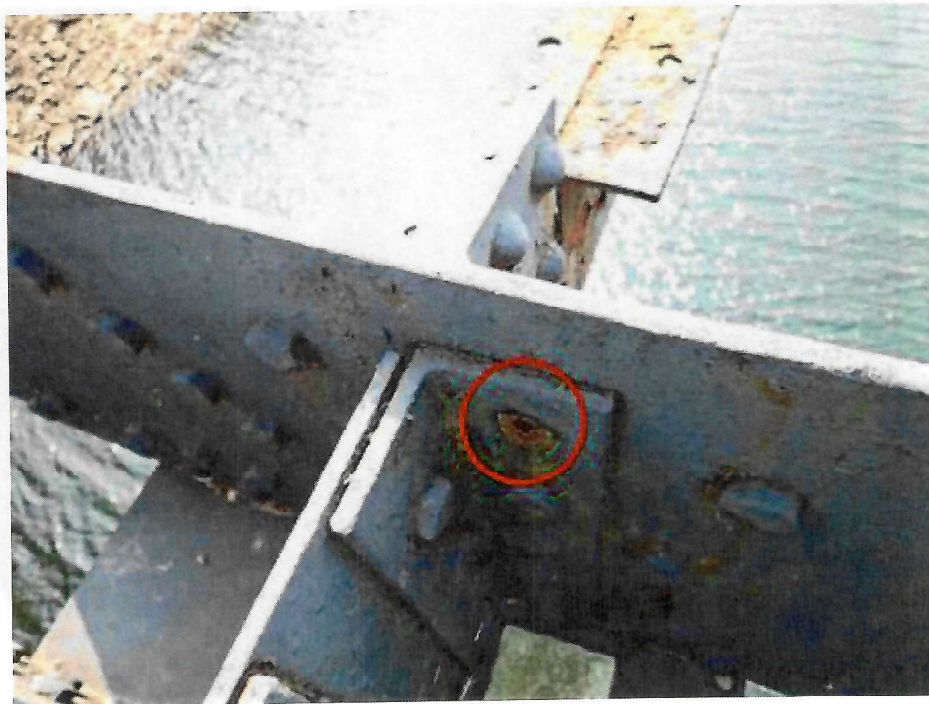
Photo 22: South Outer Truss, Outer Gusset Plate Diaphragm Angle - Sheared off connection bolt head
