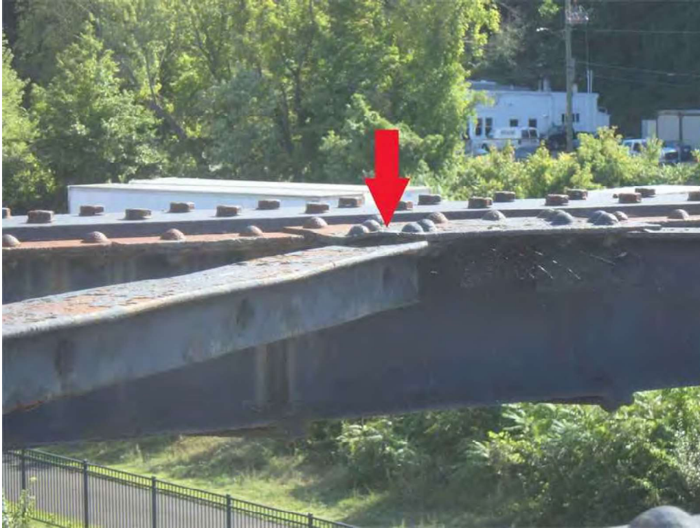
Photo 33: North tower outer truss, member U12-U14 lateral bracing connection plate - pack rust and minor bends.
