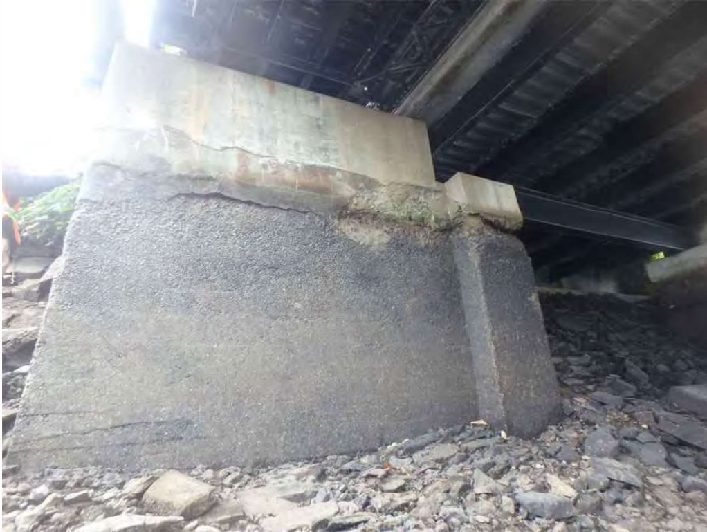
Photo 41: Northeast pier, west face – at the normal water line are spalls and hollow areas.
