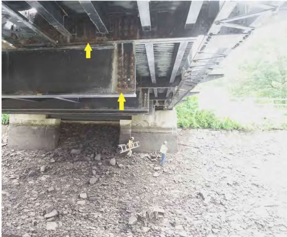
Photo 25: Span 2, floorbeam 6, west face at the south end - sidewalk floorbeam has moderate rust; roadway floorbeam has light rust. Note the connection bolts and nuts with moderate rust.
