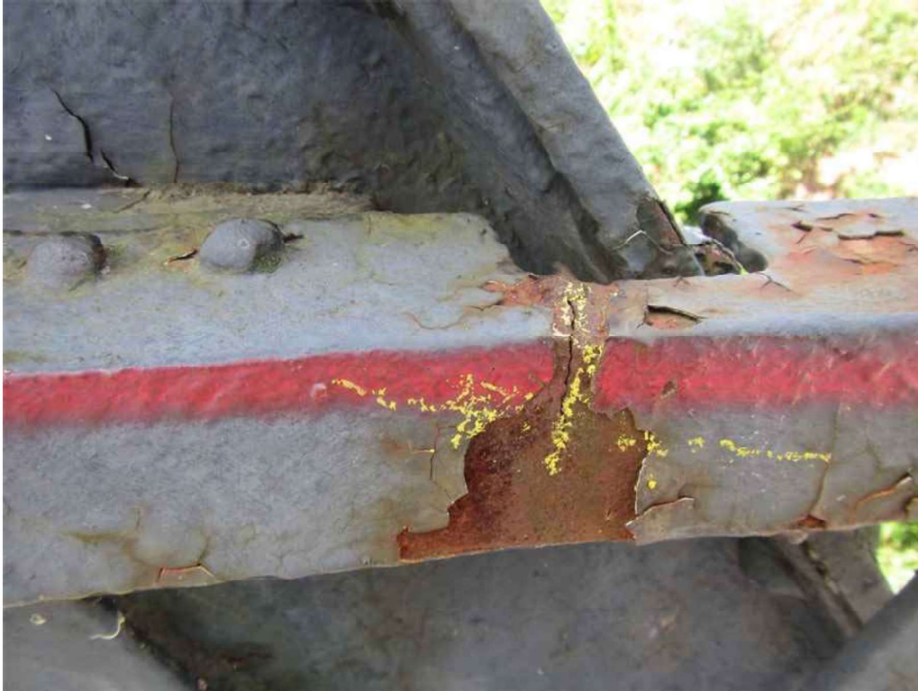
Photo 17: South sidewalk pedestrian railing, top rail, at L0-U1 - at the cut-out section is a transverse crack.
