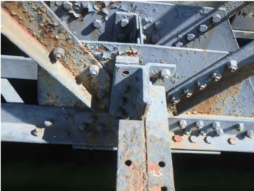
Photo 34: South tower outer truss at node L10: the diaphragm angle connection (also serves as outer connection angle for the utility support bracket) has a sheared / missing connection bolt.
