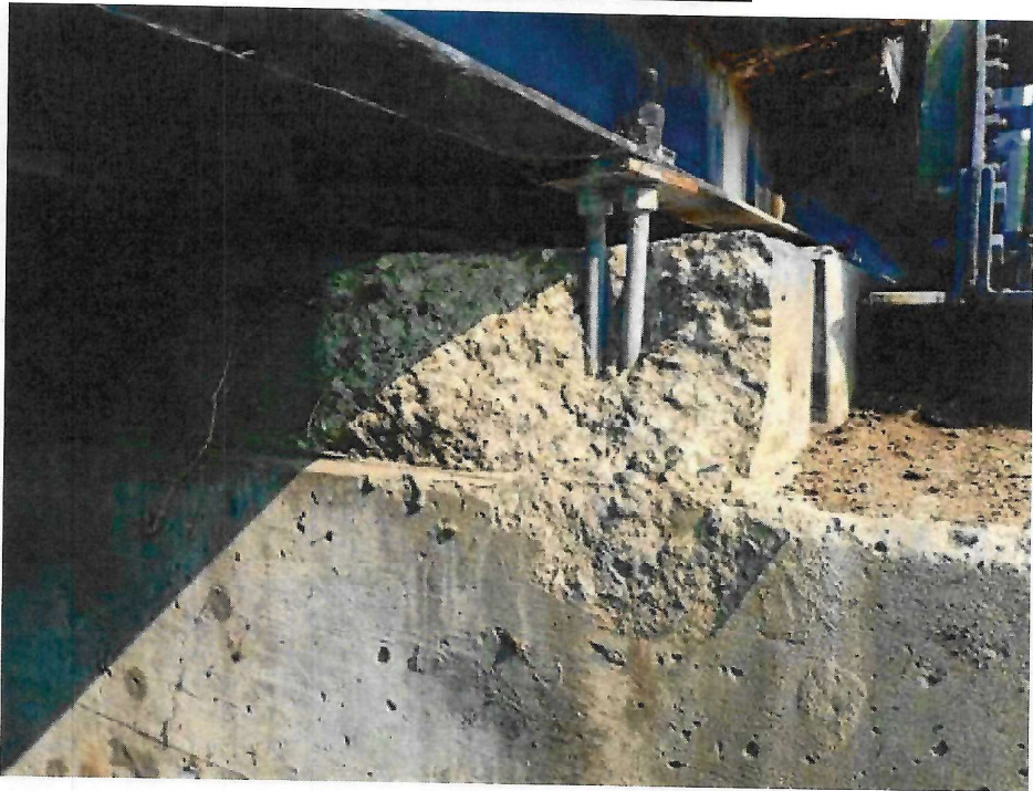
Photo 27: Southwest Pier Sidewalk Stringer Pedestal, West Face, at SW 8 - spall exposing the anchor rods and undermining the masonry plate
