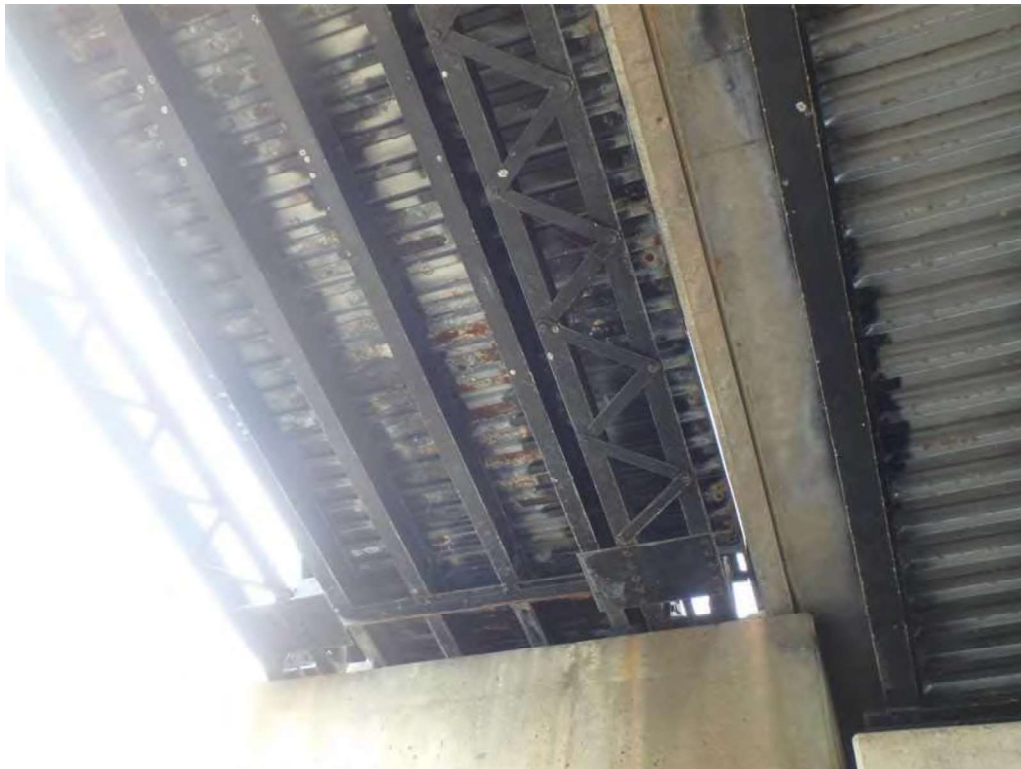
Photo 8: SIP forms, underside of south sidewalk, span 2, panel 1 (between floorbeams 1 and 2), near the southwest pier, looking west - moderate to heavy corrosion.
