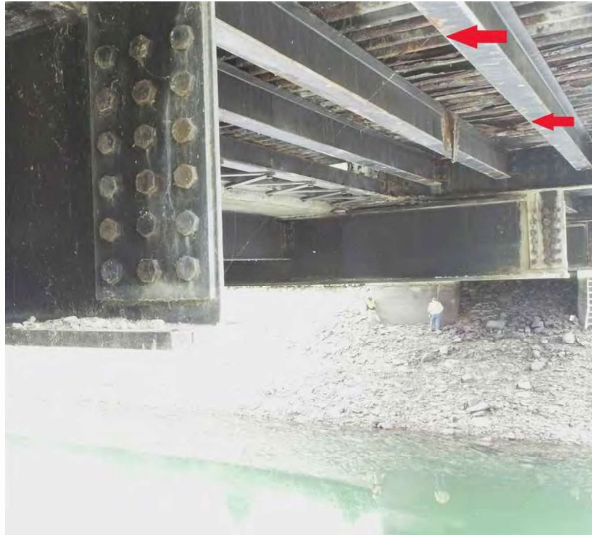
Photo 9: SIP forms, underside of south sidewalk in span 2, panel 2 (between floorbeams 2 and 3), looking east - heavy rust with isolated holes and heavy efflorescence leakage.
