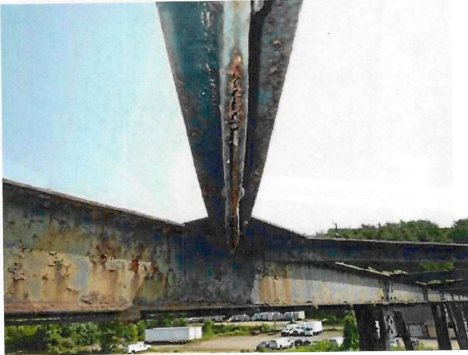
Photo 21: South Truss – pack rust between the lateral bracing angles
