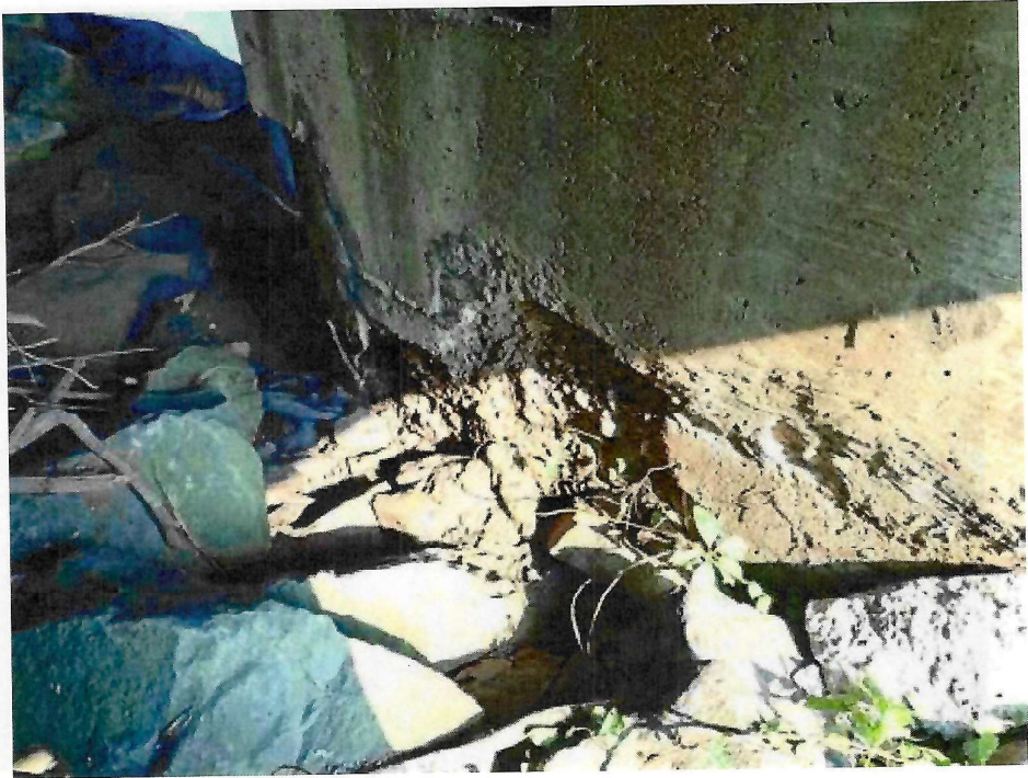
Photo 29: Southwest Pier, West Face – Spall near the rip-rap
