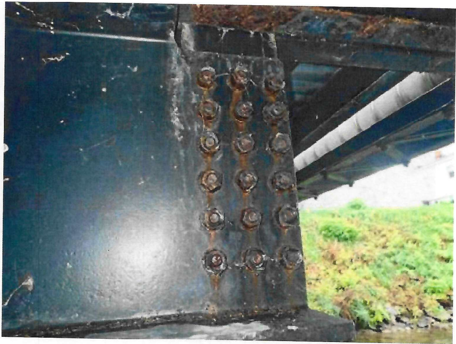
Photo 16: Roadway floorbeam to sidewalk floorbeam connection bolts with rust
