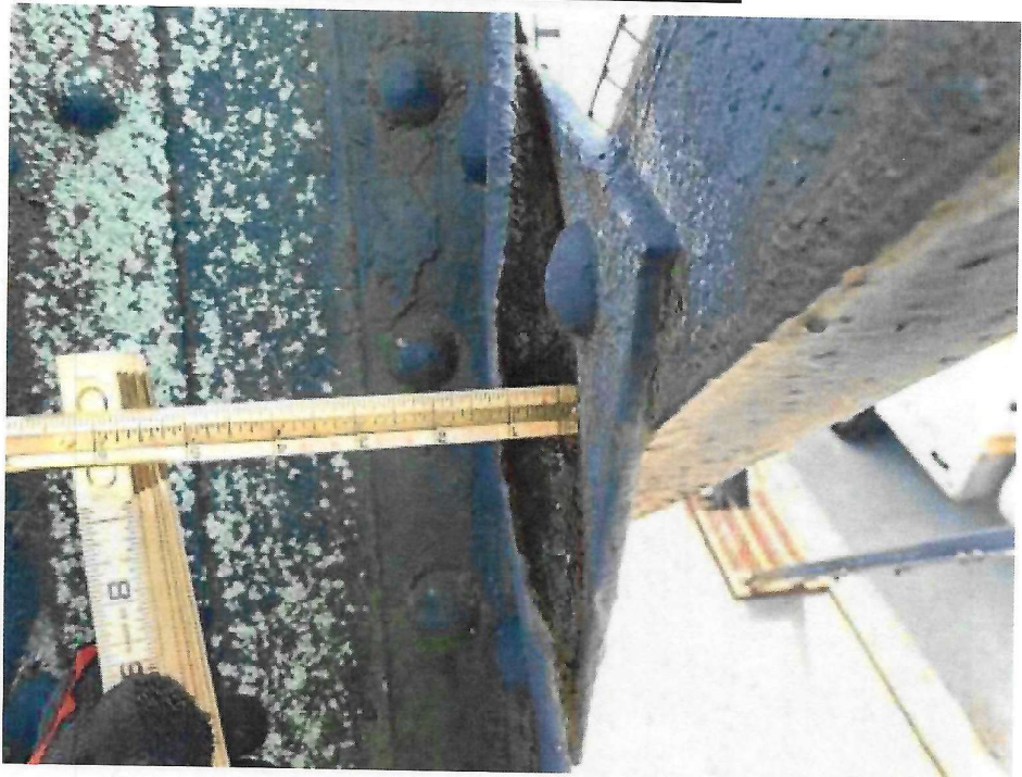
Photo 19: North Outer Truss, U8-L6 at M7 – pack rust and flange section loss
