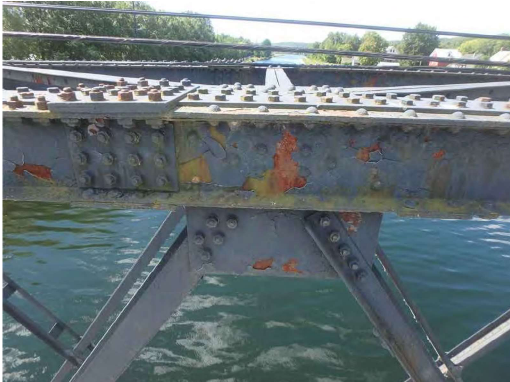
Photo 26: South tower inner truss at U12 – upper chord, lateral bracing and gusset plates with peeling paint and light rust.
