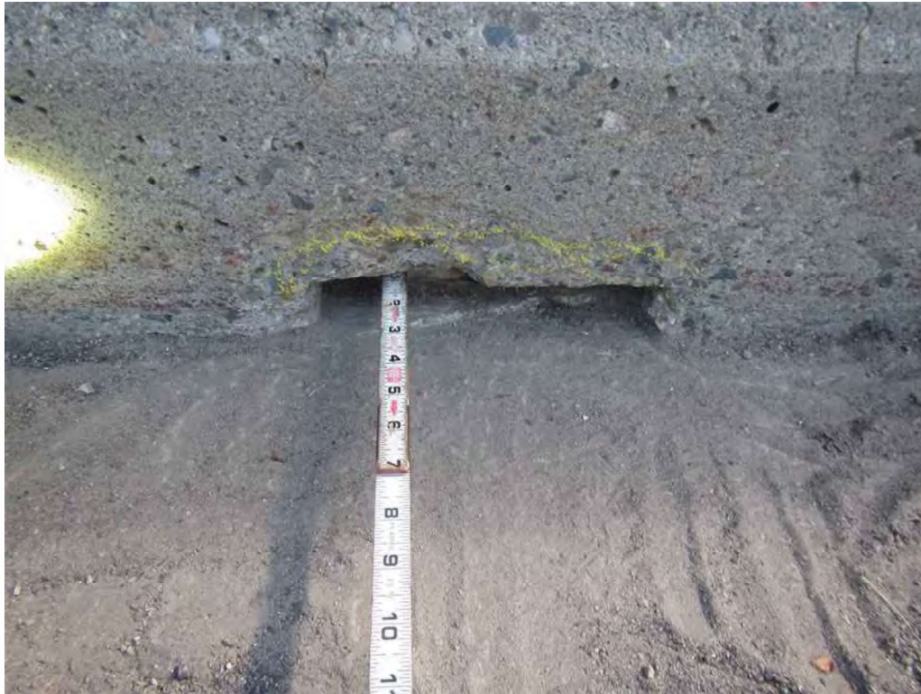
Photo 13: North curb, span 2, near L18, looking north – spall.
