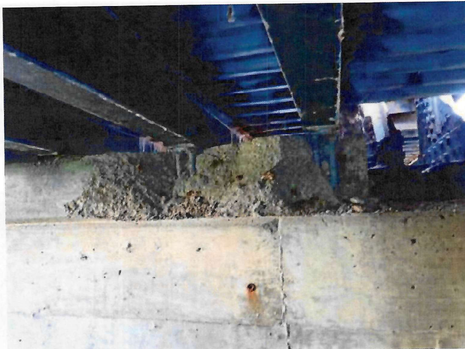
Photo 26: Northwest Pier Sidewalk Stringer Pedestal, west face, at SW3 and S4 - spall exposing the anchor bolts and undermining the masonry plate
