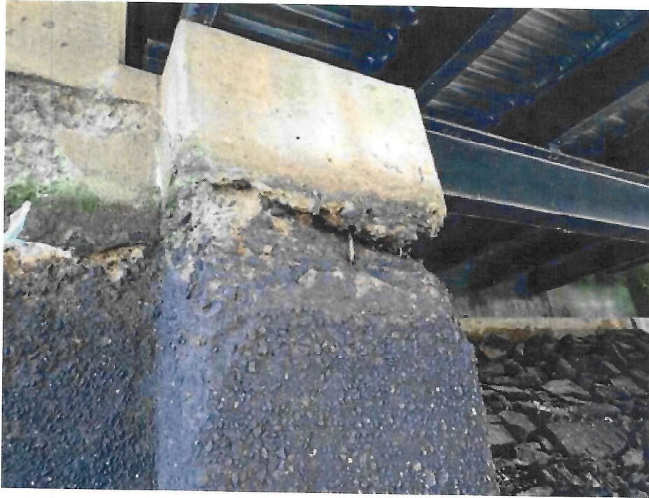
Photo 31: Northeast Pier, West Face, South End – Spall at the normal water line extending into the north extension
