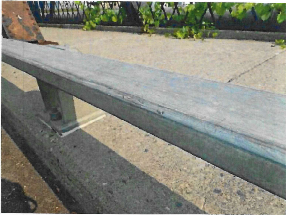
Photo 8: BR-2 Bridge Rail, Northeast Corner - scrapes and gouges
