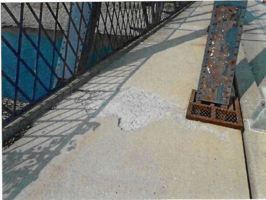
Photo 6: South Sidewalk, at L18 - spall along transverse joint
