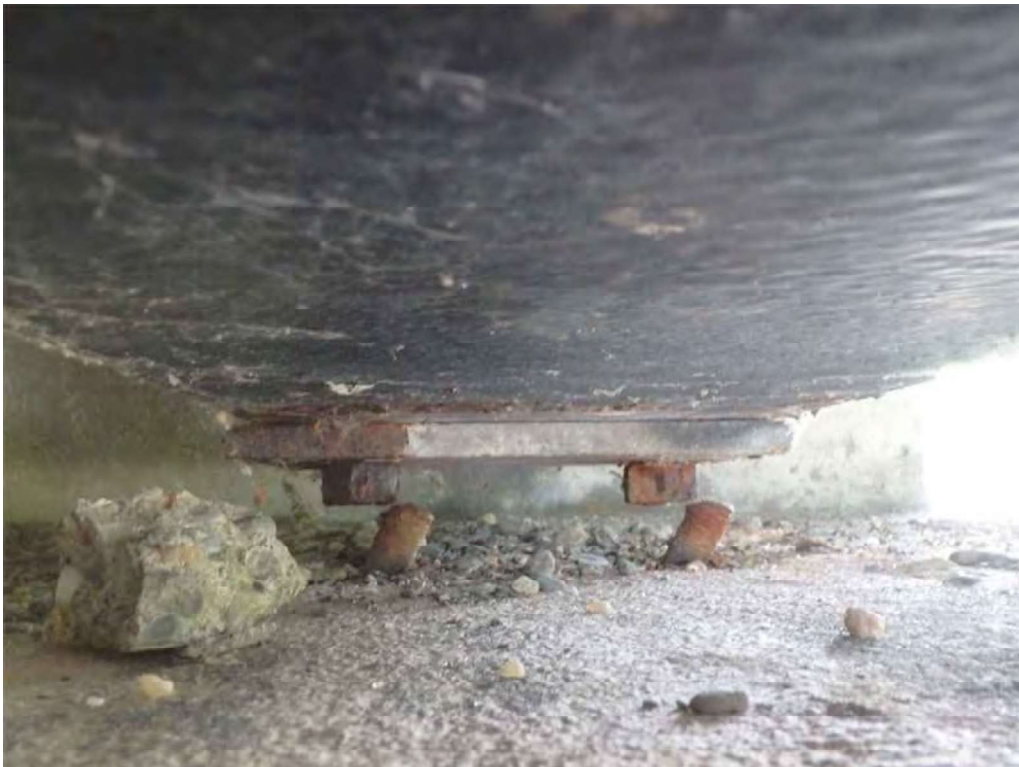
Photo 36: Northwest pier, at floorbeam 1 - both anchor rods are sheared and the floorbeam is unsupported. Note the completely spalled pedestal.
