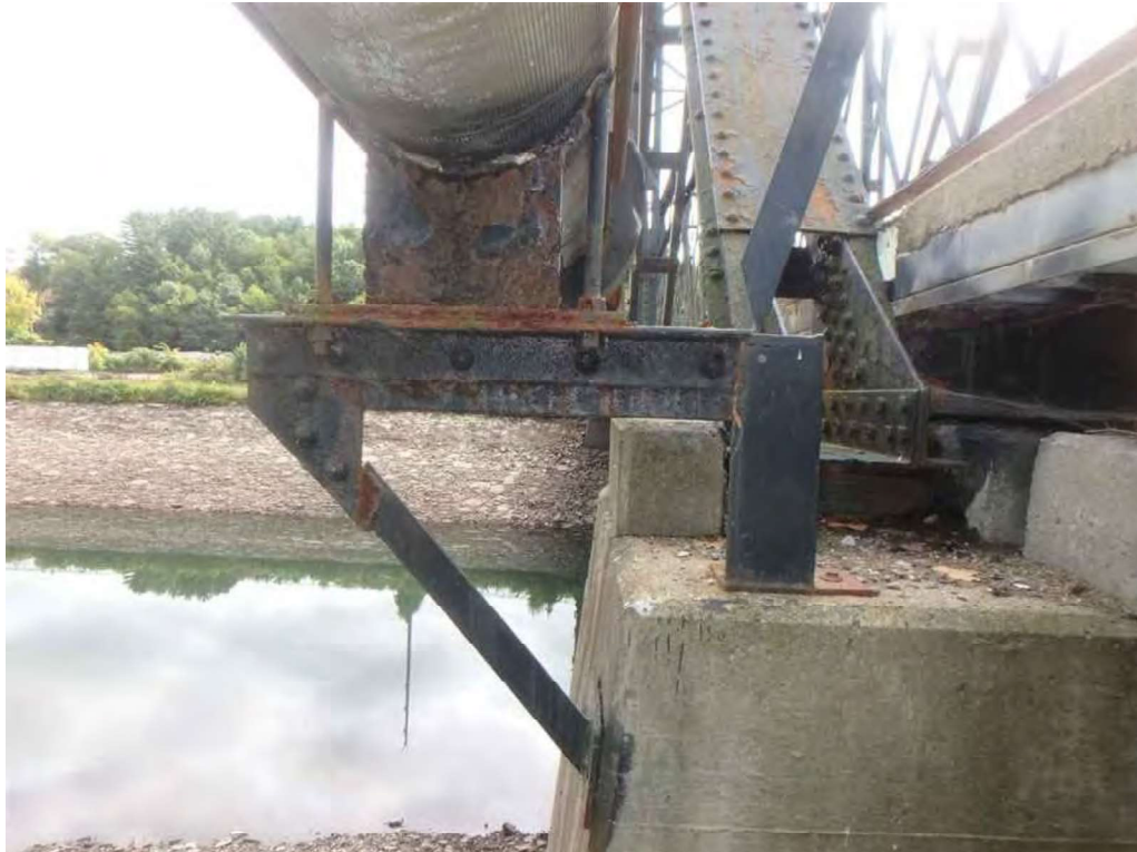
Photo 20: Steel utility support at the northwest pier, looking east - peeling paint and moderate rust.
