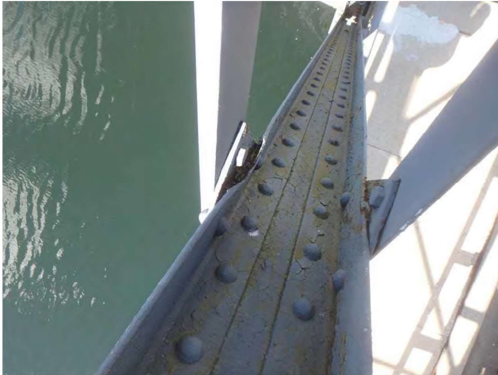
Photo 31: South tower inner truss, members U4-L2 at M3 – outer flange has section loss at the edge.
