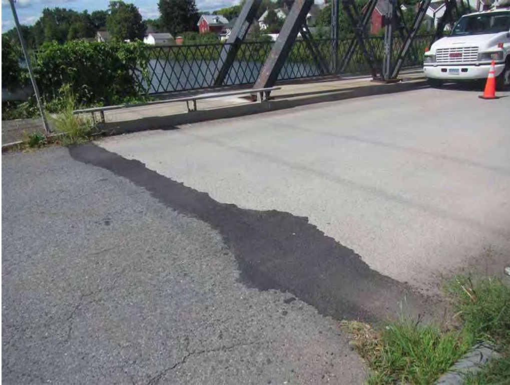
Photo 21: East abutment and bridge deck interface, looking southwest - bituminous repair patch.
