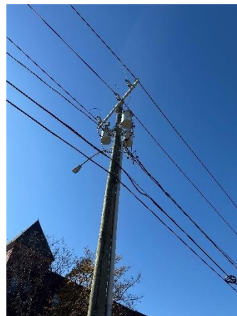
Three (3) pole-mounted electric transformers observed near southern corner of Subject Property, at the corner of Second Street and Avenue A. No petroleum releases were observed on transformers or on ground surface immediately below.
