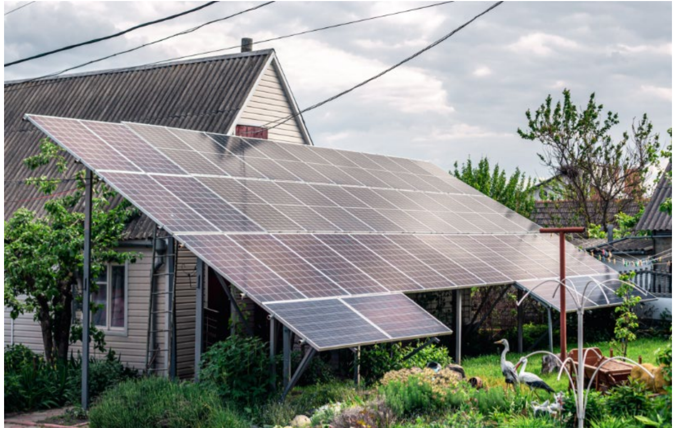
Image of an approximately 20 kW ground-mounted solar system next a small home. Photo credit: ASG
