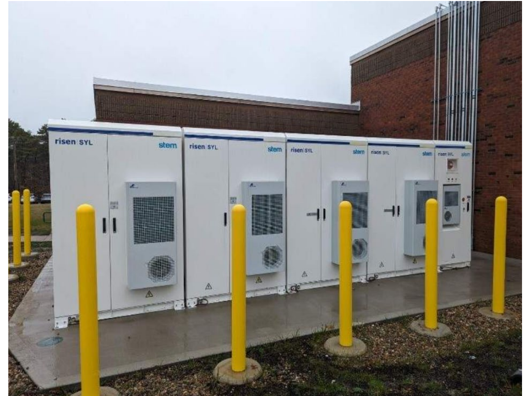
Image of a 1 MW battery storage system at the Dennis-Yarmouth Regional High School in Yarmouth, MA. Photo credit: Department of Energy Resources and CVEC
