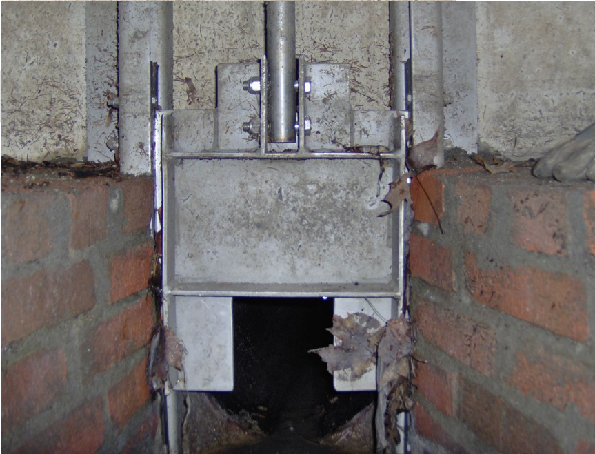
Photo #3: Avenue A Bufferline Gate Orifice Plate
