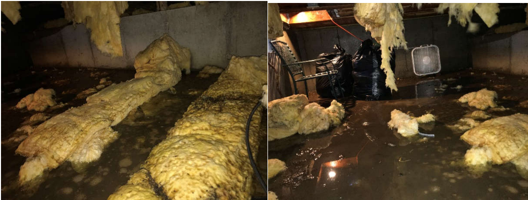
Water damage and mold in the concrete section of the basement from the most recent rat incident when they chewed through the water line in the refrigerator.
