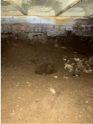
Rat tunnels in the dirt floor of the basement
