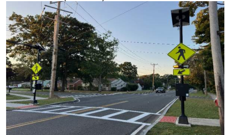
RECTANGULAR RAPID FLASHING BEACONS (RRFBs)
