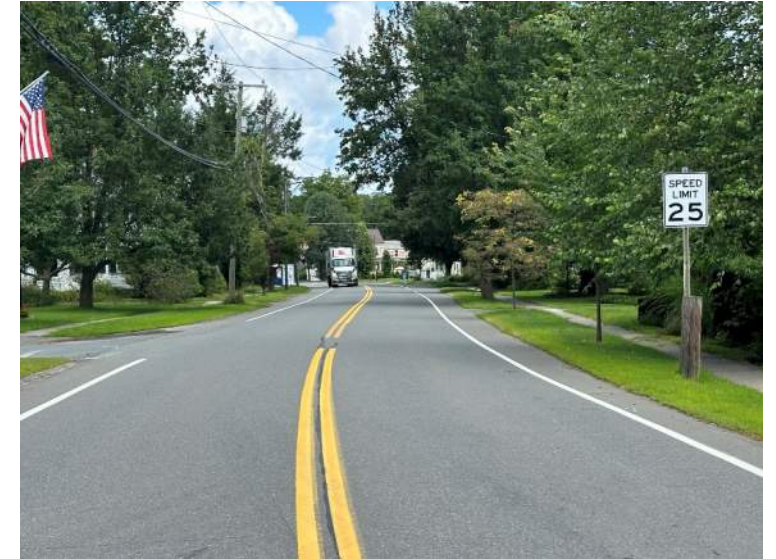
LACK OF DEDICATED BICYCLE FACILITIES
